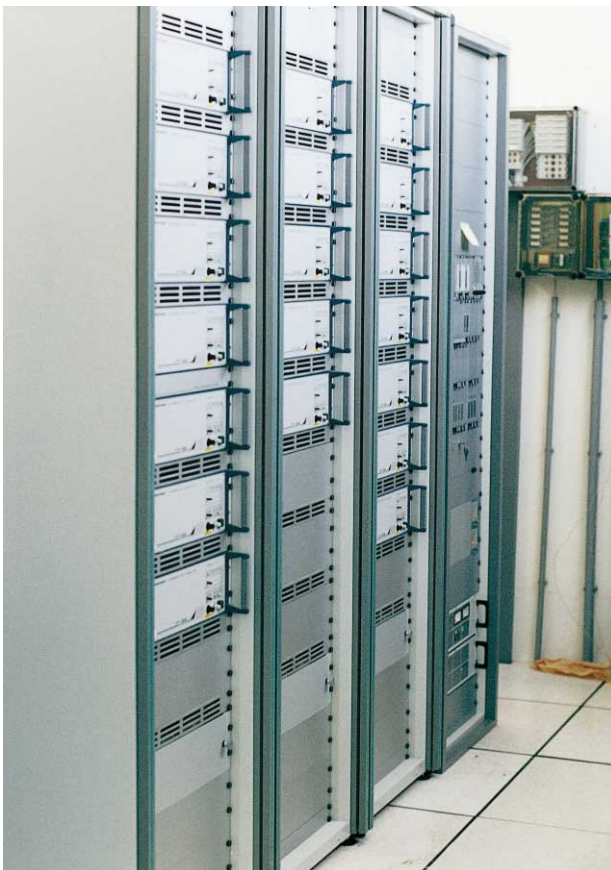
FIG 5 A glance into the North transmitting center at Vienna's Schwechat airport: series 200 wherever you look.
