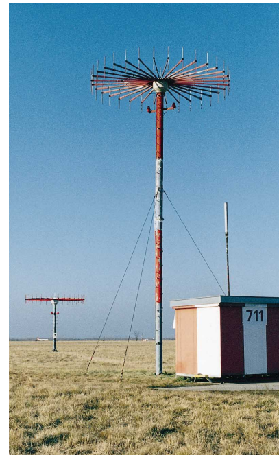
FIG 8 Two direction finders from Rohde & Schwarz at Vienna Schwechat: the old PA007, still working well after 21 years, and the new PA100
