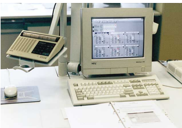
FIG 7 All receiving stations throughout Austria are monitored and operated through a telecontrol system from workstations like this one.
